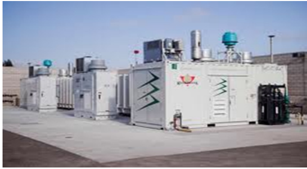
Figure 6-1. Commercial Fuel Cell for CHP Application
