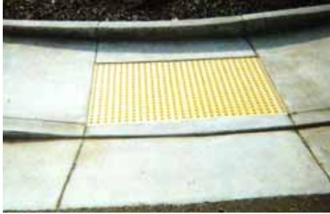
Figure 11-7. Photo. Detectable warnings treatment in Roseville, CA.
